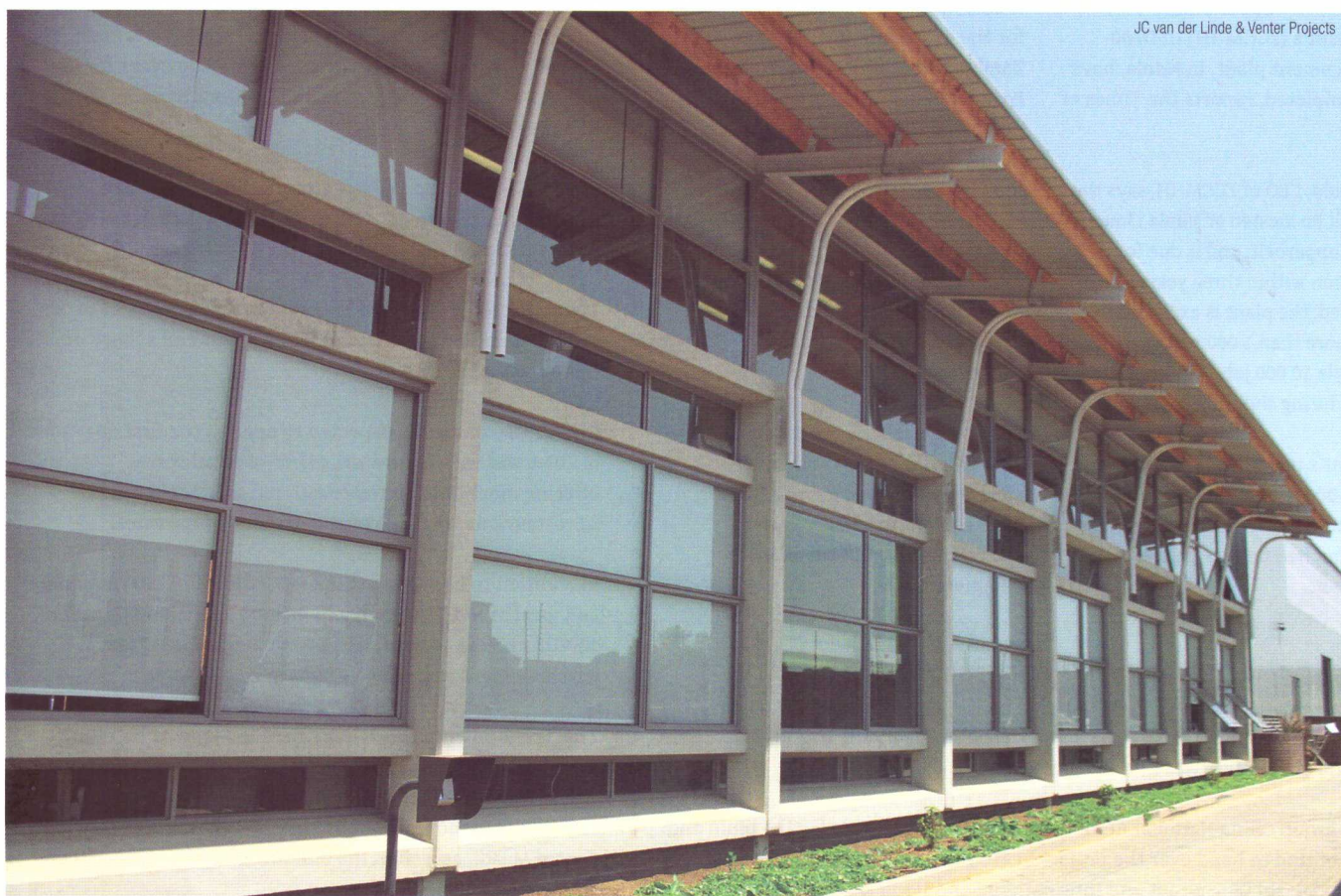
A roof overhang over the north-facing windows of the I-CAT office block shades the building during summer and partially during winter.
