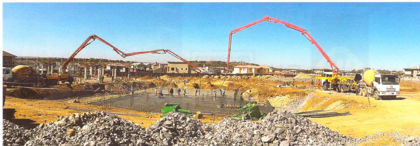
A large raft foundation was used to support one of the two new office blocks built by J.C. van der Linde & Venter Projects at
